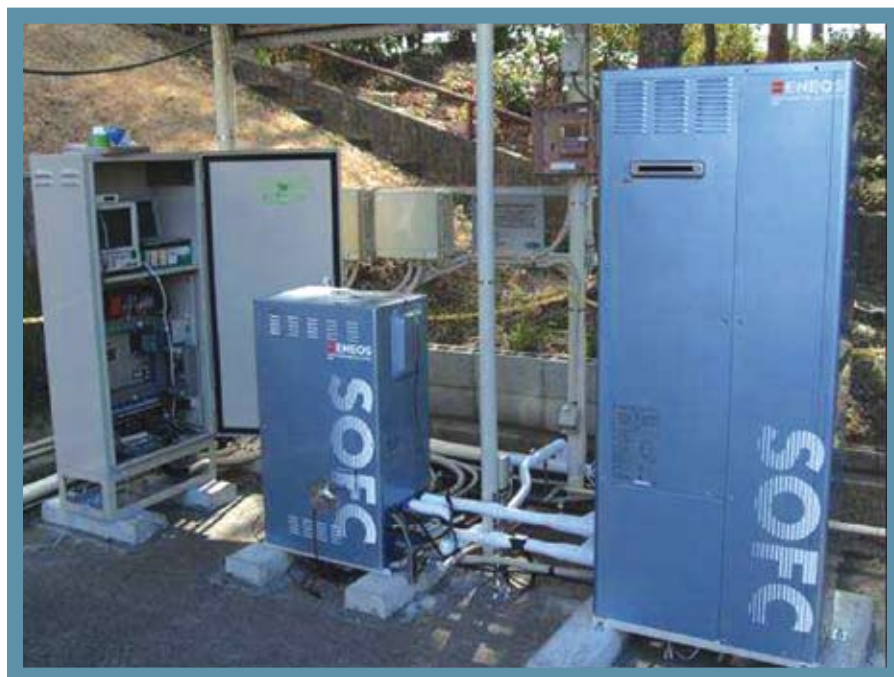
Fig. 1. SOFC-based residential CHP system showing the SOFC unit (left) and the hot water tank (right).
