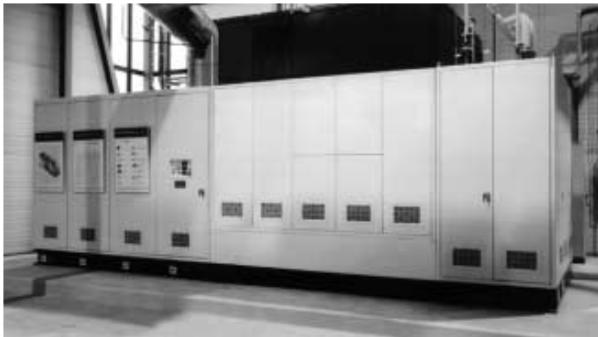
Fig. 5. Siemens Westinghouse 100 kW SOFC system installed in The Netherlands.
